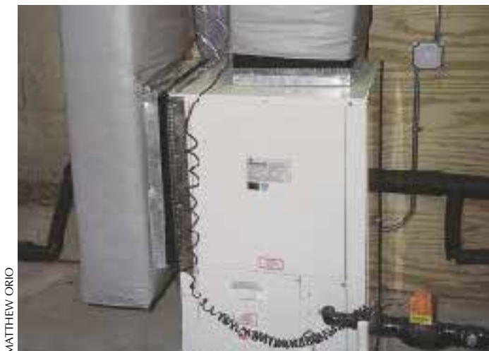
Figure 9. The ductwork for this heat-pump installation has been carefully insulated.
